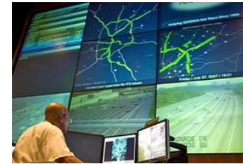
GDOT Transportation Management Centers
